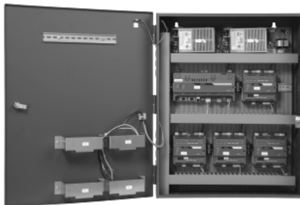
Figure 1: Security Control Panel Mounted in a 24 in. x 30 in. Enclosure
