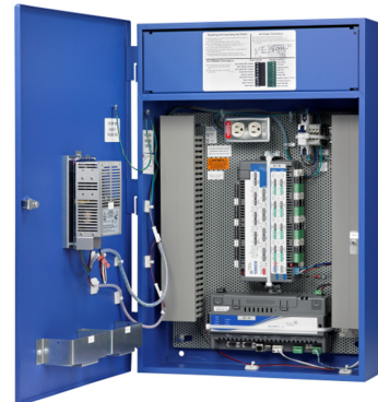
Figure 1: Security Control Panel Mounted in a 20 in. x 30 in. Enclosure
